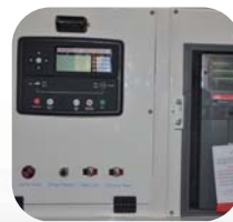
Control Panel & MCB
